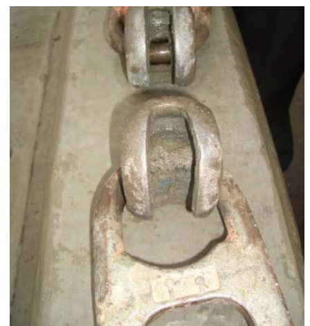
Bent, worn slot
