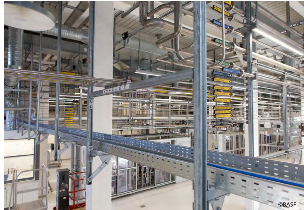
HALFEN Powerclick used as a standardized support system for all utility systems in BASF's new Research Centre M400.
