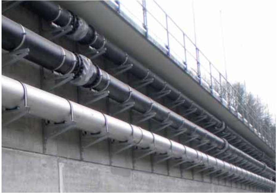
Pipe supports with cantilevers brackets in a sewage treatment plant
