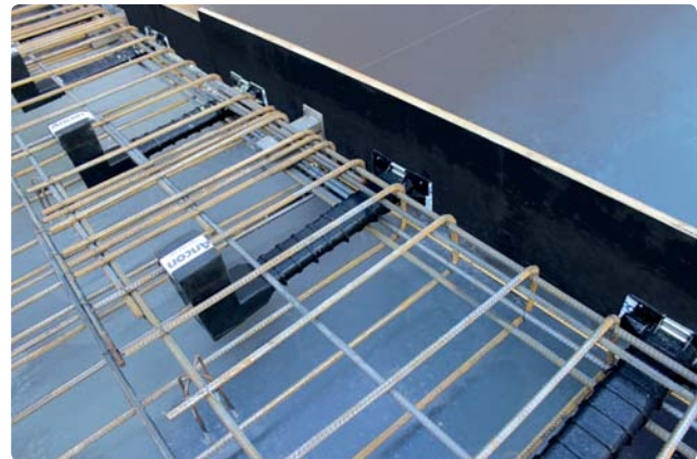
Ancon Locking Pin Sleeve, fixed to formwork.
