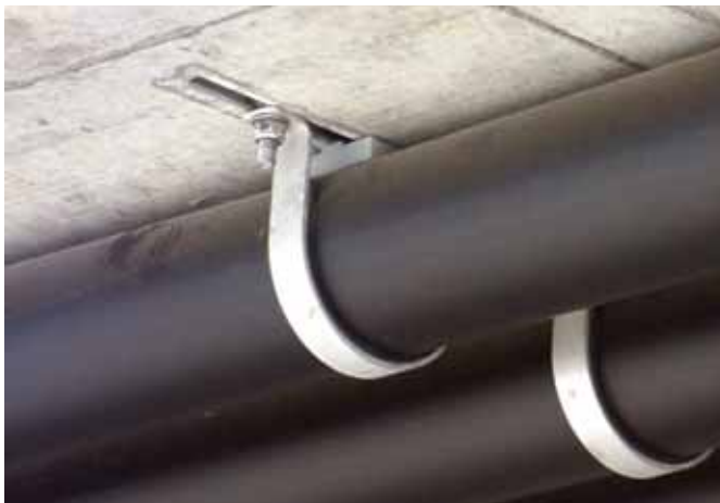
Pipe fixed to anchor channels cast into a ceiling slab
