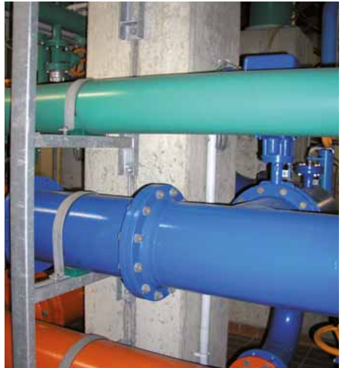
Pipe support fixed to vertical cast-in serrated channel
