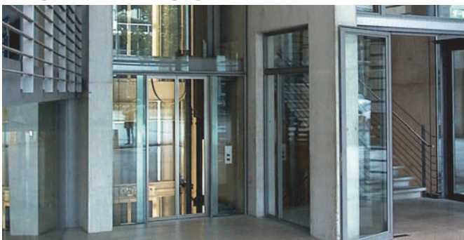
Lift fixings, guide-rails
