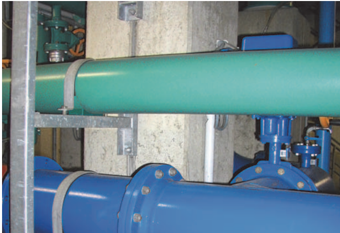
Pipe supports on vertical HZA Channels
