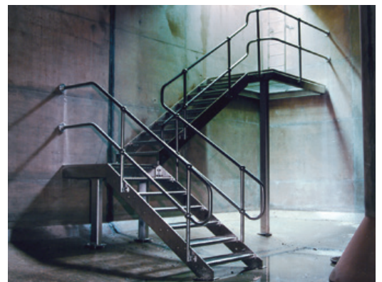
Access Walkways and Ladders
