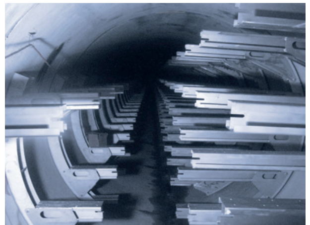
Project: Carlton Cable Tunnel, Australia (Client: Energy Australia, Contractor: The Abergeldie Group, Cable Support Engineering: Leviat)
