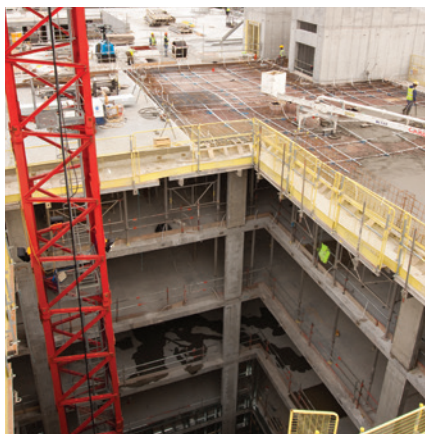
500 Lockable dowels were installed on the Emergency Care Centre in Aberdeen, UK
