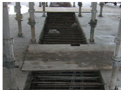
Pour Strips restrict site access, cause a trip hazard and delay progress on site
