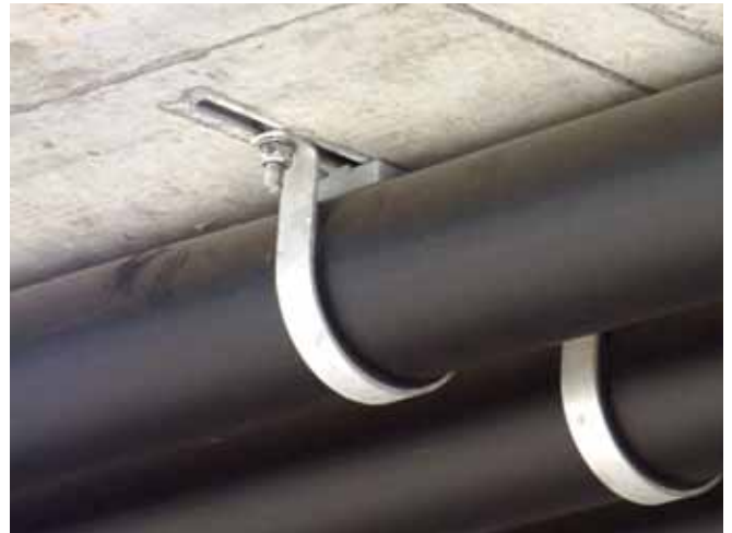
Pipe support bolted to ceiling
