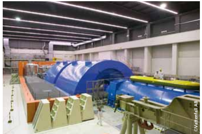
Turbine hall in nuclear power plant
