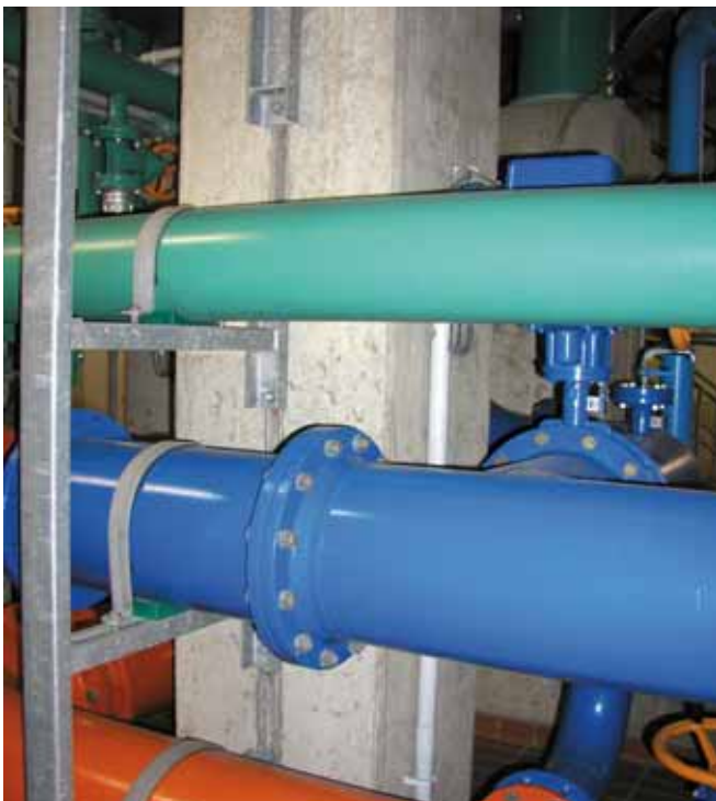
Pipe support using vertical channel
