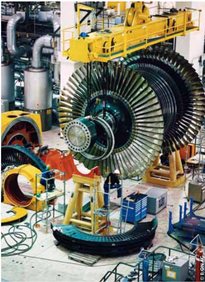
Turbine in nuclear power plant
